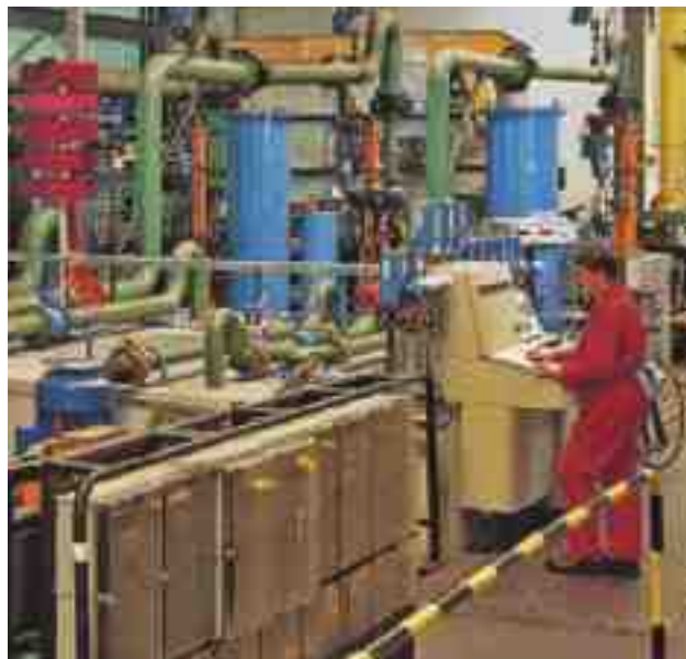
Test bed SPX Flow Technology in Assen, the Netherlands
